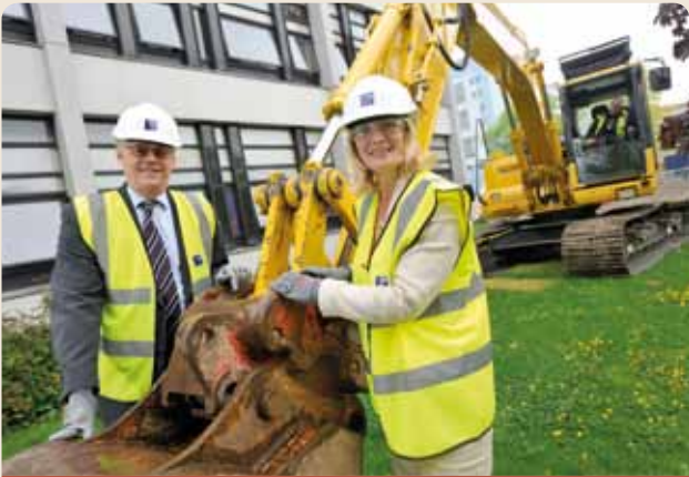
£6m new build for School of Health Studies begins: work on the site began after the Vice-Chancellor, Professor Mark Cleary, and Dean of the School, Shirley Congdon, met to cut the turf back. The School of Health Studies will be moving to city campus in Autumn 2011.
